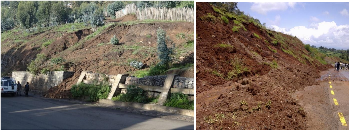
Figure 8: Sliding of Silty clay soil within constructed structure in the study road segment
