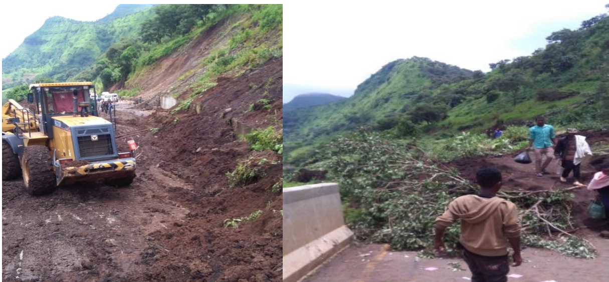
Figure 6: Slope failure(landslide) in the road segments (in Kar Mountain site)
