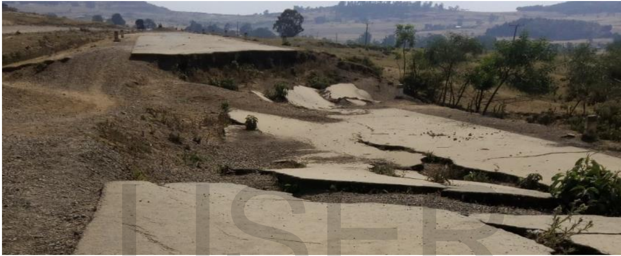
Figure 13: Model 3- road failures due to instability of slope presentation diagram
