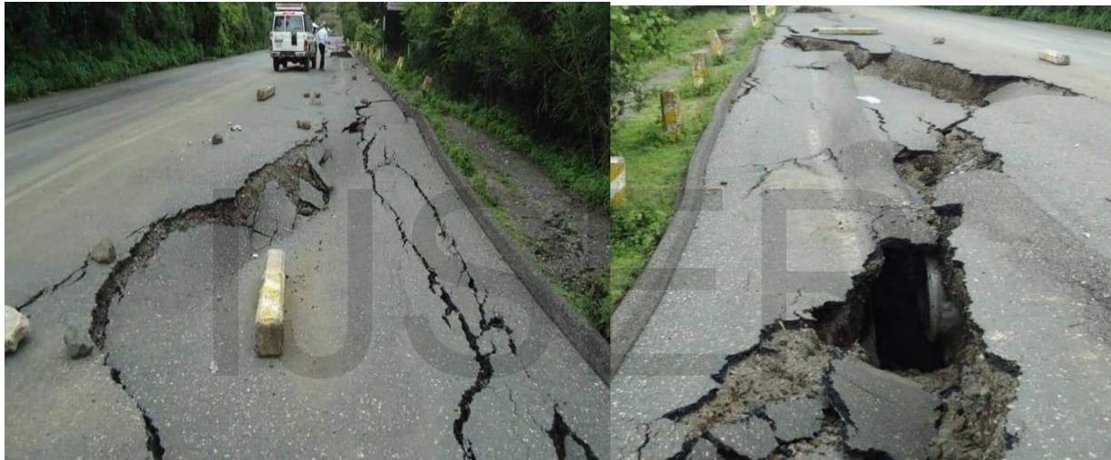
Figure 12: Model 2- road failures due to instability of slope presentation diagram and images
