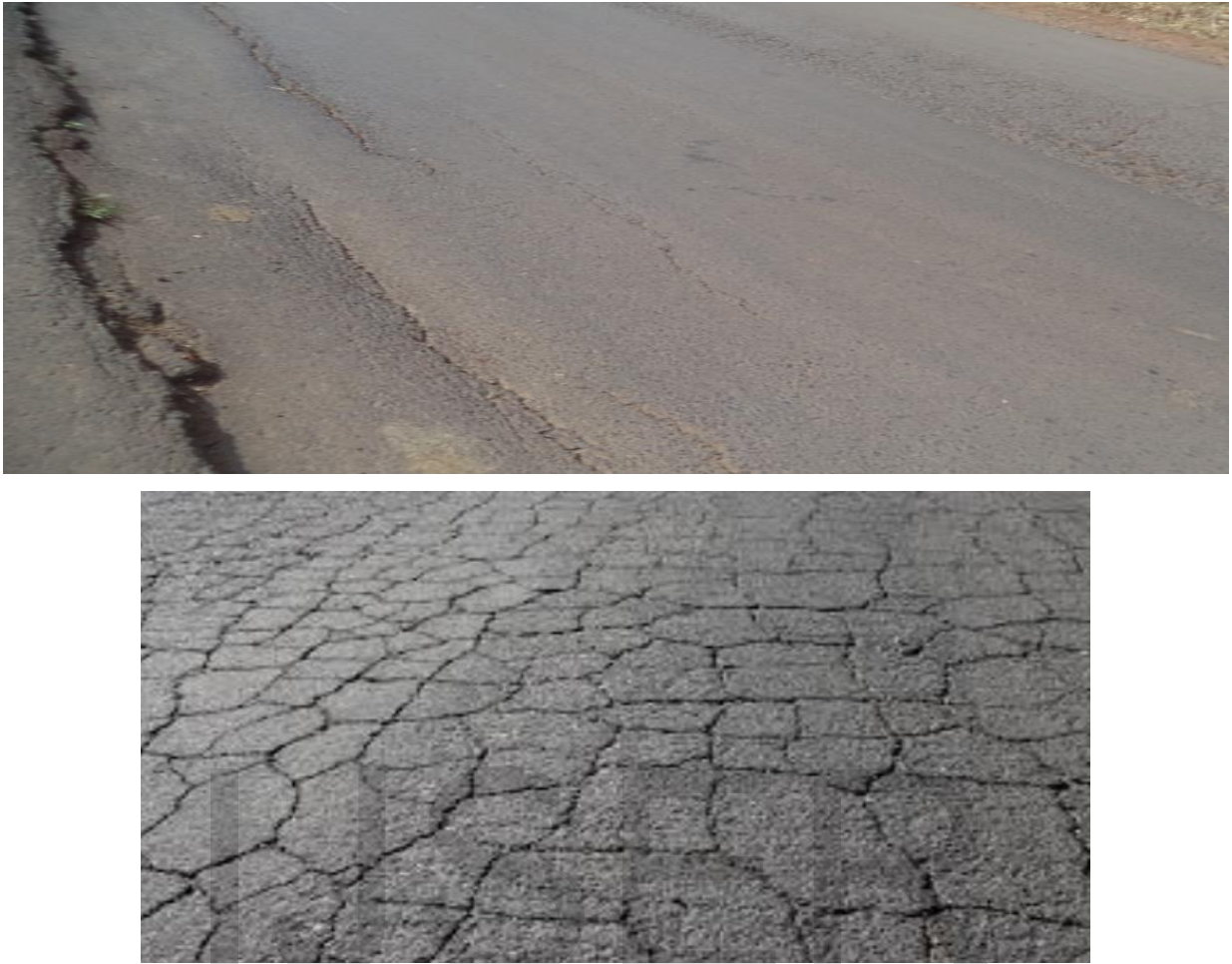
Figure 2: Expansive soil problems that causes the road failure - Cracks on the road
