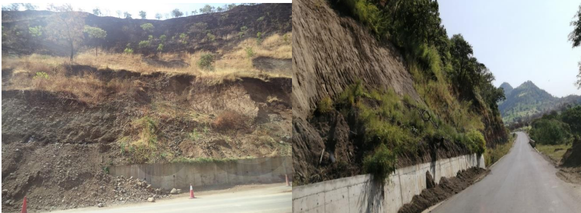
Figure 5: soil slope instability problems (Chagni – Mandura Road Section)
